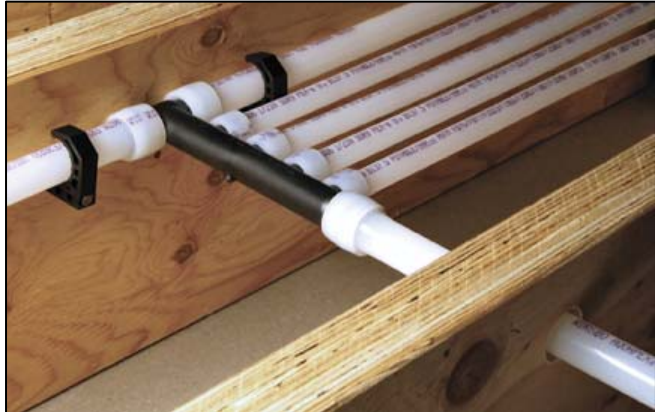
EIR: The adoption of PEX tubing into the California Plumbing Code would be “an environmentally superior action with respect to public health and hazards, water quality and air quality.”
